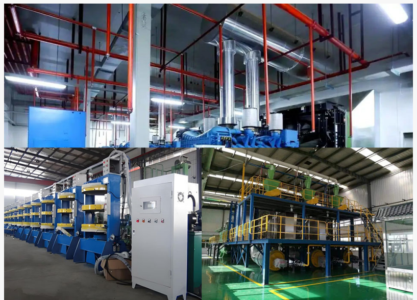
ENERZIP backup power generator equipment supports essential factory operations at LIBLIK Tires during utility power interruptions.
