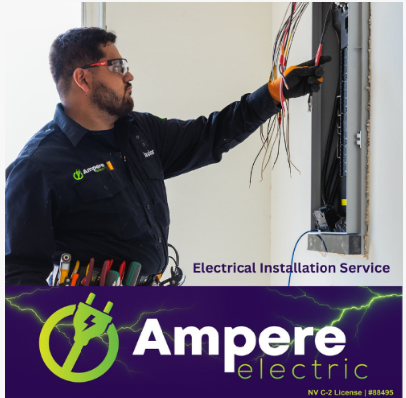
Ampere Electric Las Vegas - Electrical Installation Service
