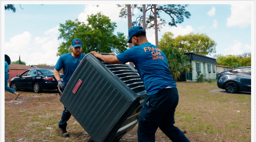
Frank Gay Services donates and installs a new HVAC unit for a local family through the Pathways to Home program.
