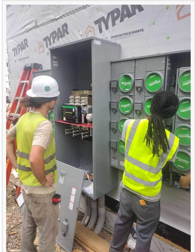
Industrial Electrical Services.
