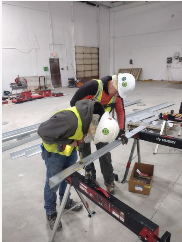
Commercial Electrical Contractors.
