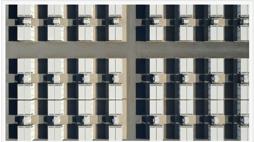
Aerial view of the Prevalon HD5™ AC integrated battery energy storage platform showcasing a high-density utility-scale site layout designed for scalable deployment, optimized constructability, and long-term operational performance.
