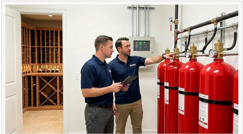
Expert inspection of a Clean Agent Fire Suppression System
