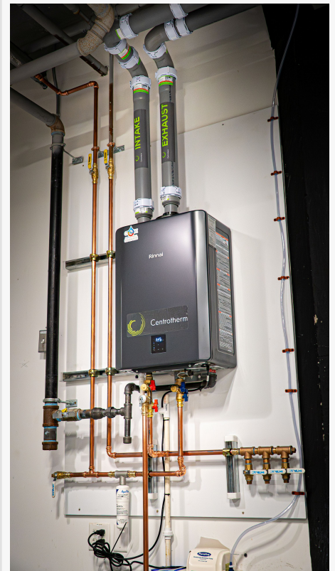
Rinnai Boiler with Centrotherm Venting
