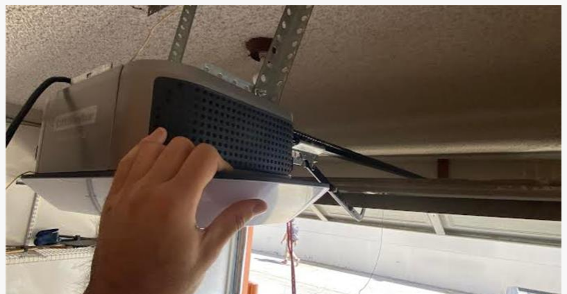
Garage door cable repair and inspection service for Pasadena homeowners experiencing uneven or stuck garage doors.
