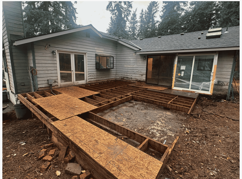
Deck Renovation Before
