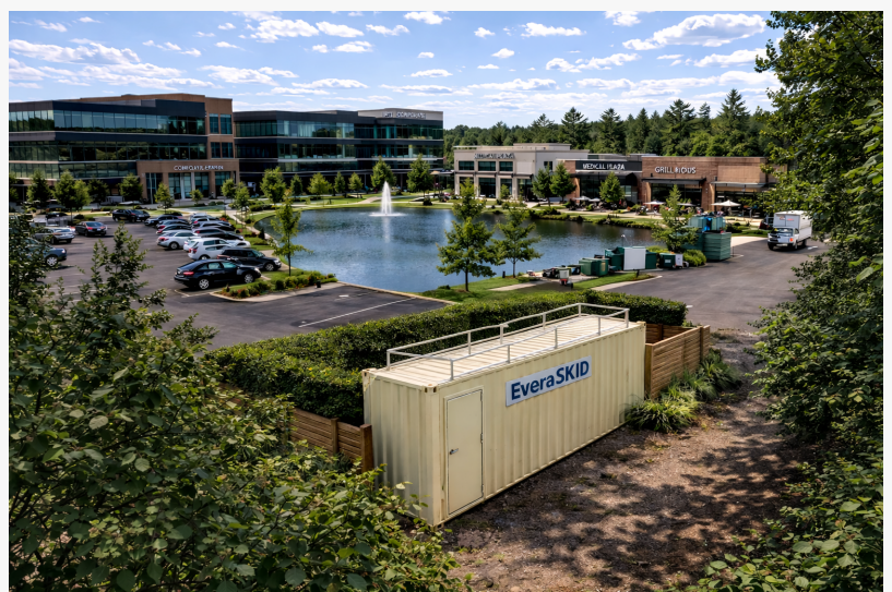
Representative treatment facility installed at a commercial site.
