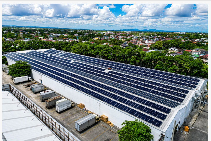
Aerial view of Liwayway Marketing Corporation's Oishi facility in Imus, Cavite, featuring a large-scale rooftop solar PV installation by Solaren Renewable Energy Solutions Corp. to help reduce electricity costs and support cleaner operations.
