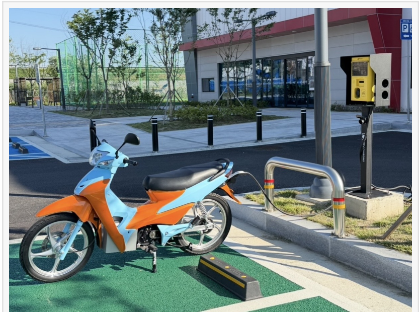
charging from standard EV charging station
