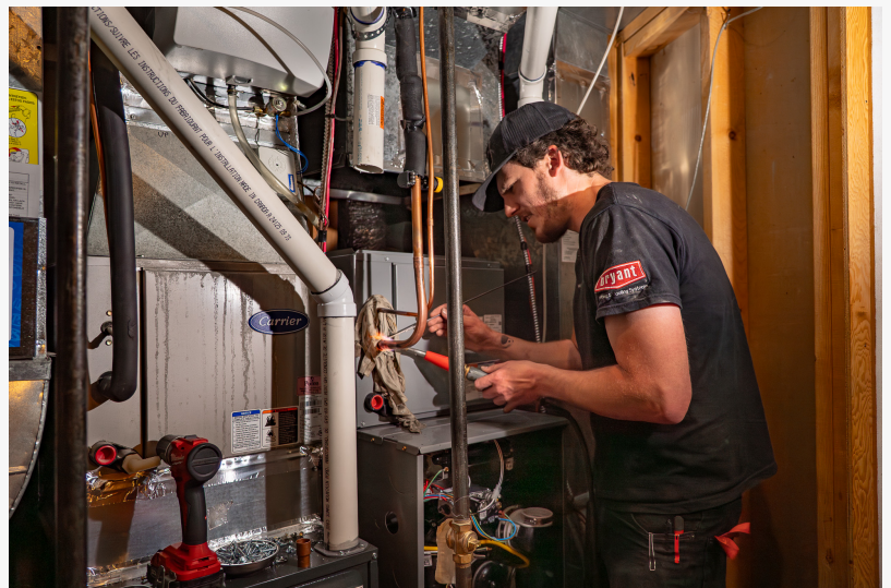
Furnace Installation Service
