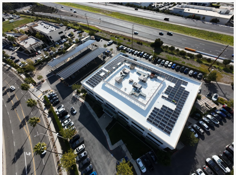
300kW rooftop and carport solar drone photo
