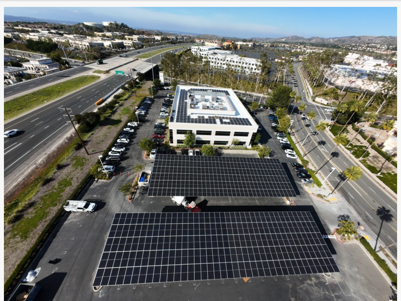
300kW rooftop and carport commercial solar
