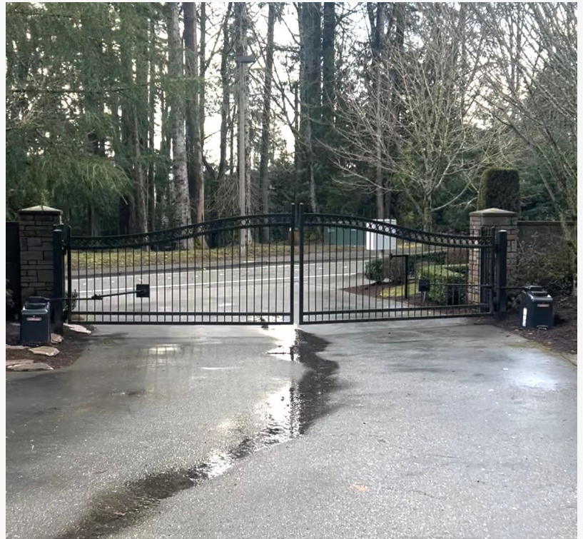
Full HOA gate installation with access control management
