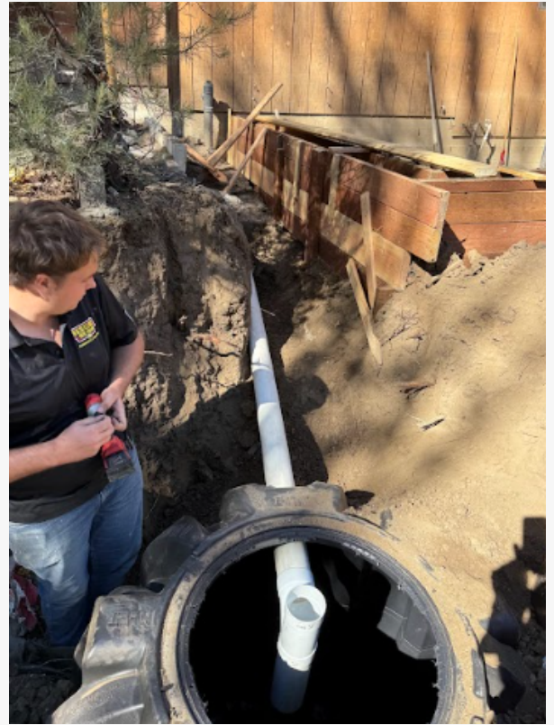
Professional infrastructure solutions and sewer repair to keep your property compliant and functional.
