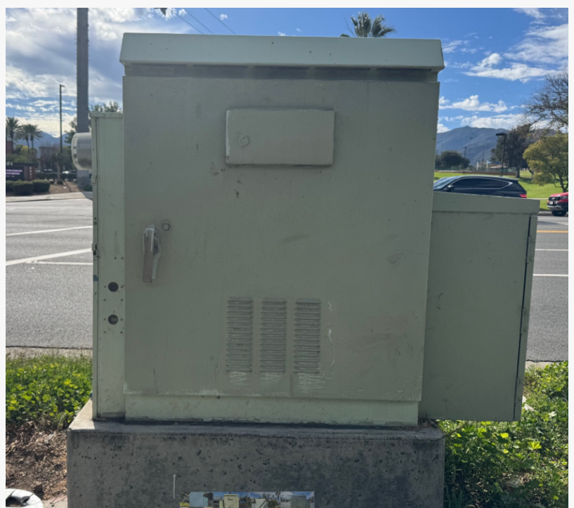
Utility Box – Sidewalk-Facing View Before Art Wrap
