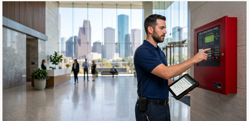
Fire Alarm System Services in Downtown Houston
