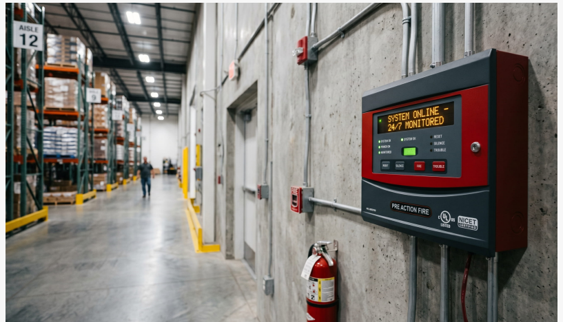
Fire Alarm Monitoring Services in Thornton, CO
