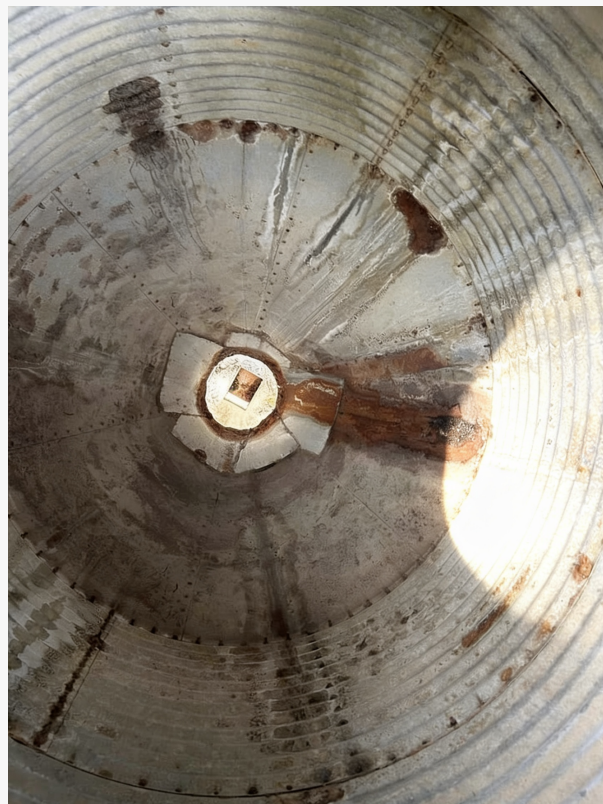
Interior view of a corrugated grain bin showing corrosion and staining before protective lining.
