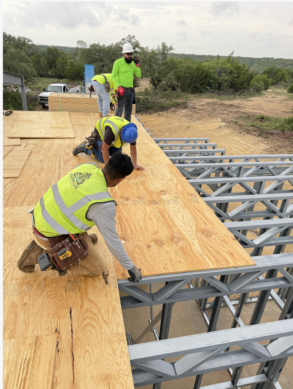
TX Sparks Constructions team members install structural components on-site, reflecting the company's focus on precision execution, steel and light gauge steel construction methods, and commercial-grade building practices.
