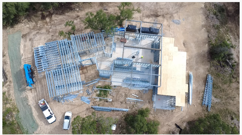
Drone view of a TX Sparks Constructions project showing active structural progress and coordinated development supported by centralized planning and technology-enabled project management.
