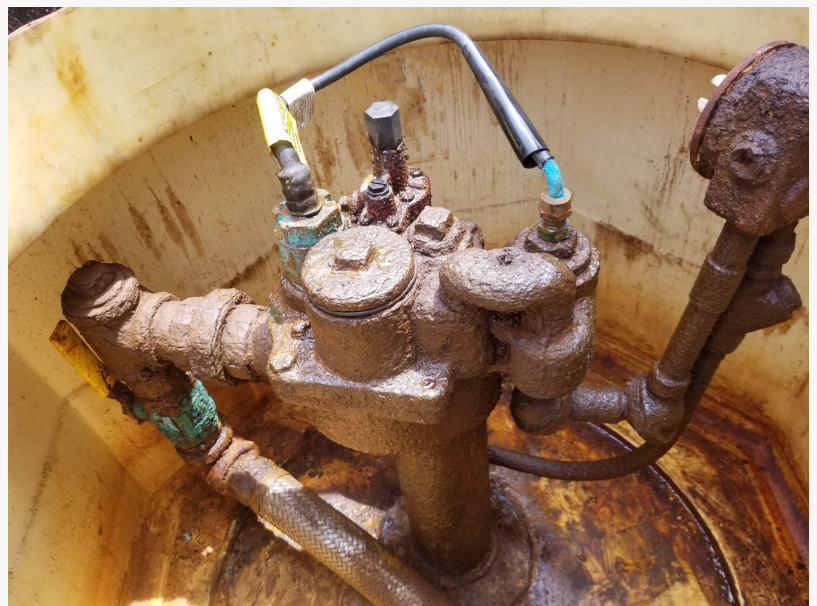
Untreated Rusty Ethanol Containment System
