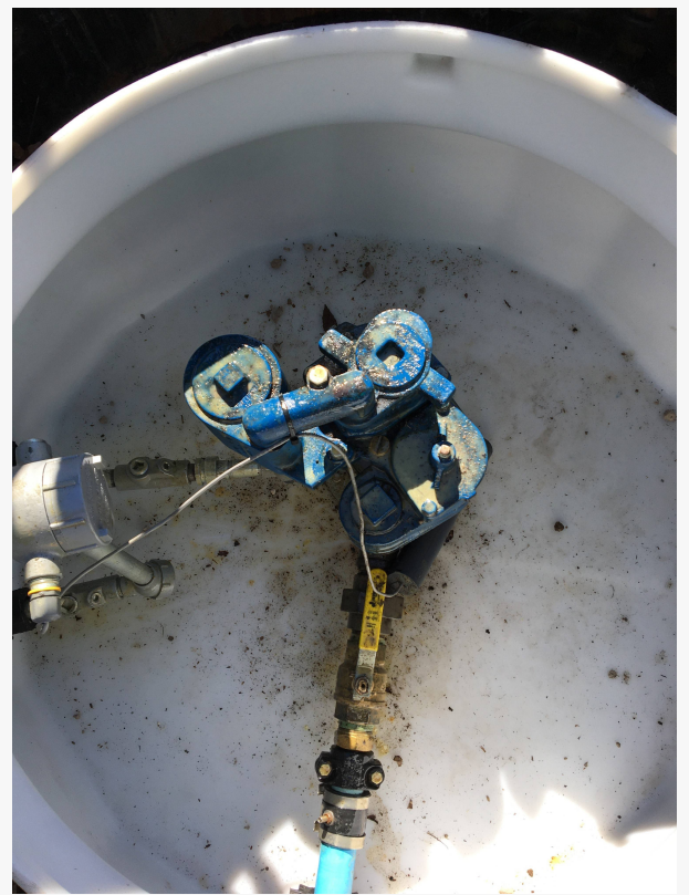
Same Ethanol Pump Treated With HinderRUST, 359 days later.
