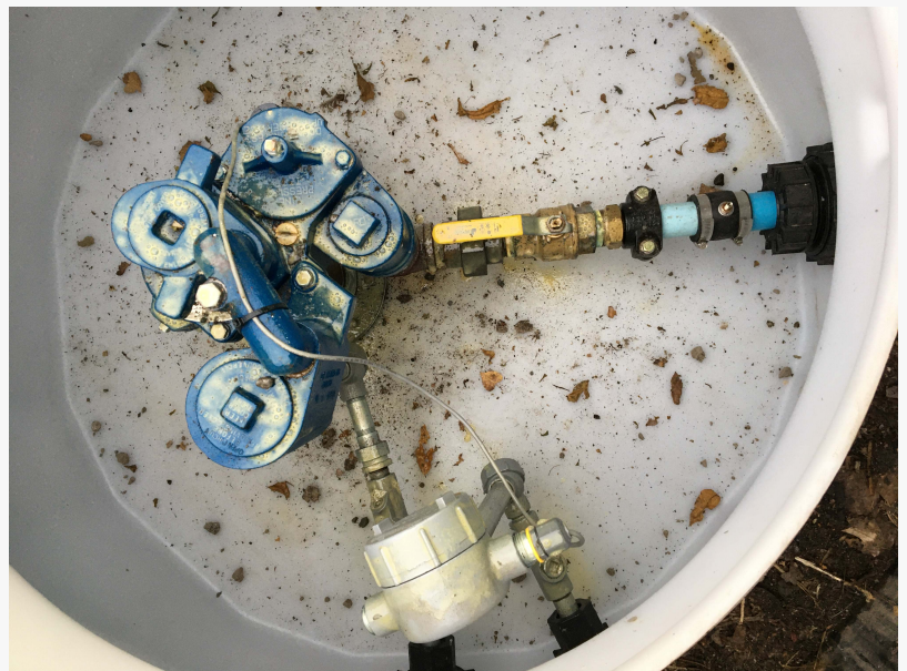
Newly Installed Ethanol Pump, Treated With HinderRUST
