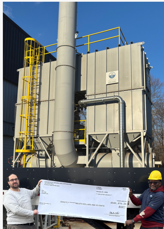
A Ship & Shore Environmental air pollution control system installed at a Connecticut Natural Gas Corporation facility represents a $560,970 savings due to emissions reduction and energy efficiency.
