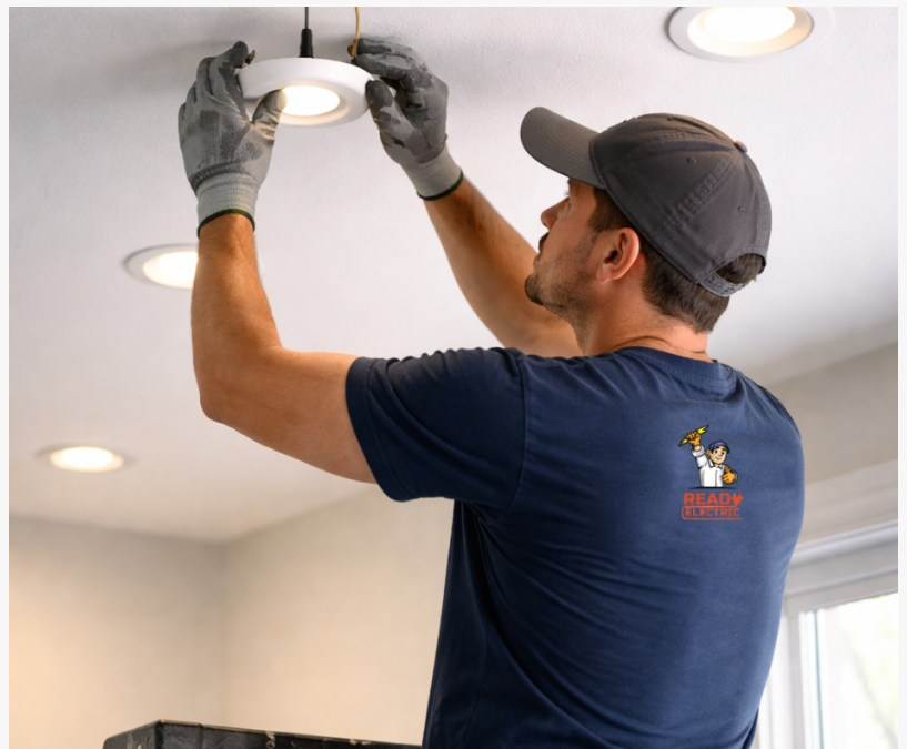
Ready Electric offers 24/7 emergency electrical repair for urgent power, breaker, outlet, and wiring issues in Los Angeles.
