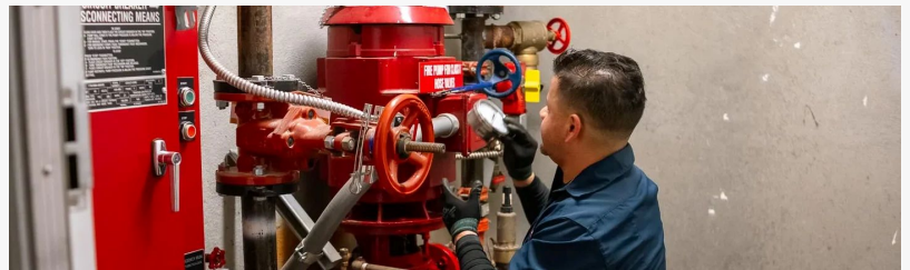
Fire pump inspection
