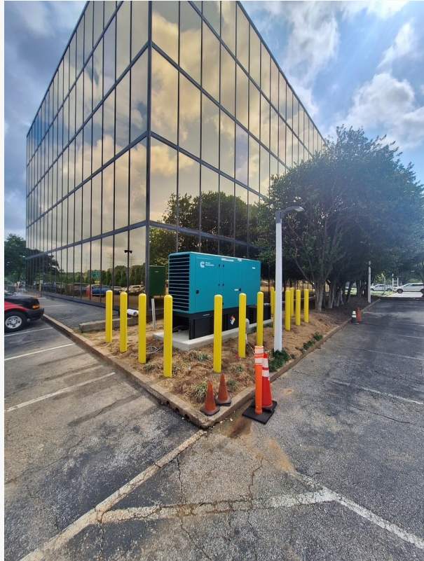
Cummins 200kW diesel generator installation by Benchmark Electric, LLC
