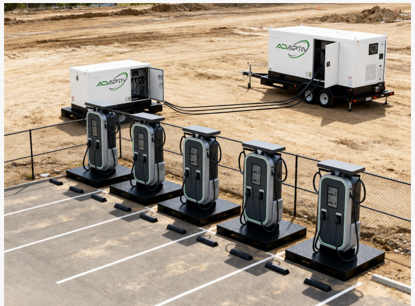
Off Grid EV Charging - CAAS
