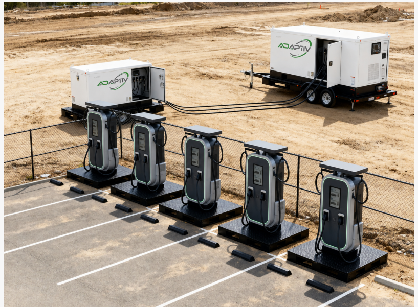
Off Grid EV Charging - CAAS
