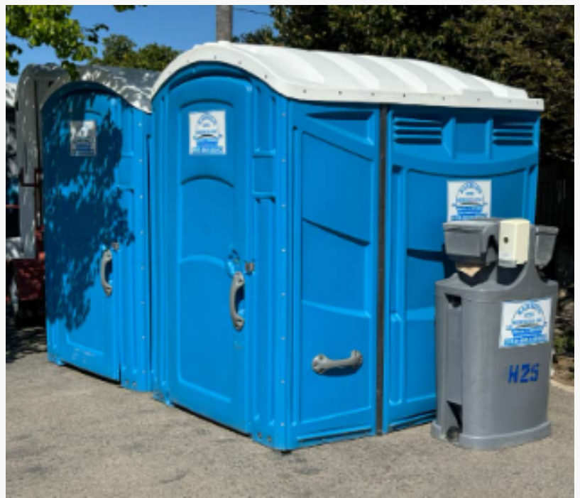
Clean portable sanitation units and a standalone handwash station from Barrios Site Services, Inc., designed to maximize construction site hygiene and labor productivity.
