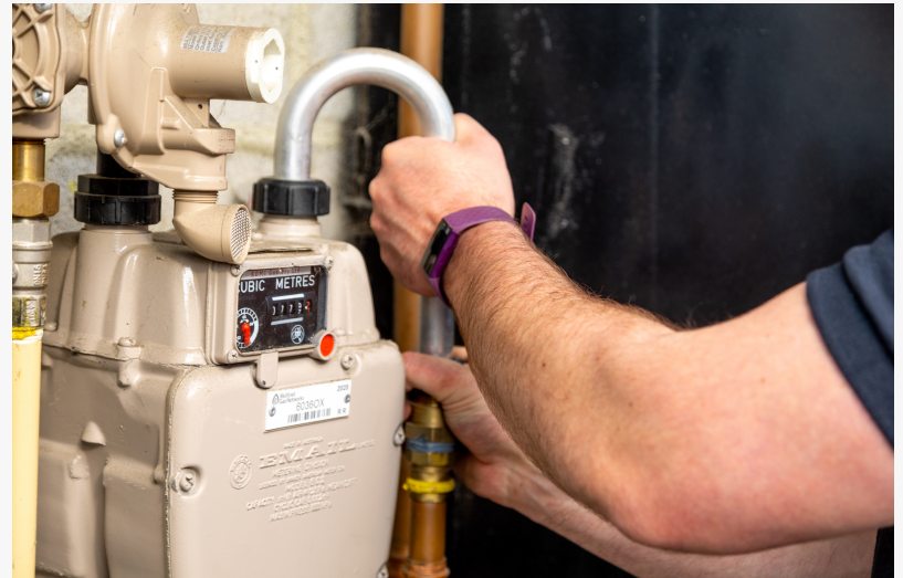
Hot water systems are among the most heavily used household appliances during winter.
