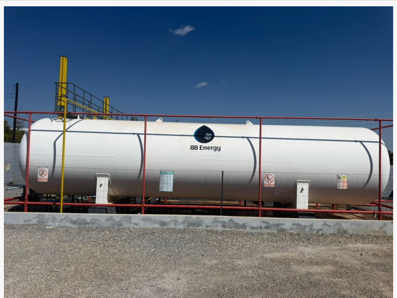
New BB Energy LPG Storage Tank in Zambia
