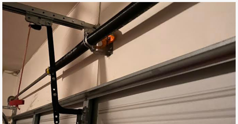
Garage door cable repair is one of the common services requested by Pasadena homeowners.
