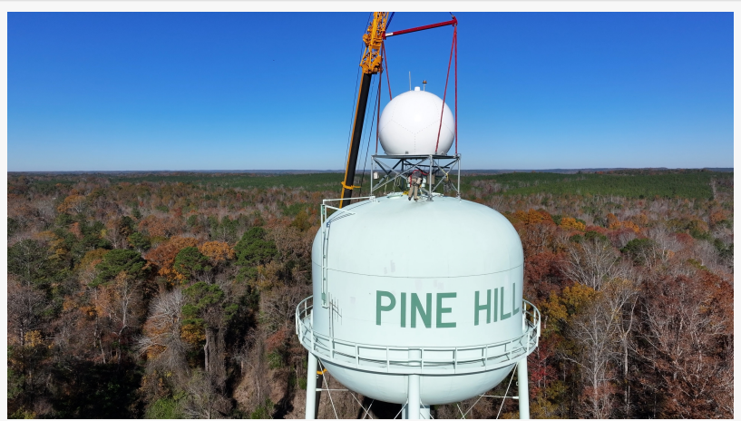
Climavision's X-band radar installed in Pine Hill, Alabama
