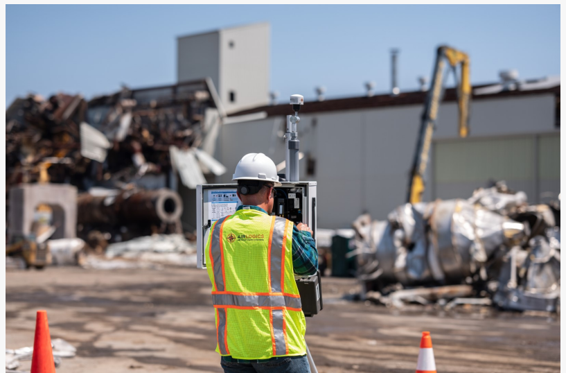
Perimeter Air Monitoring System
