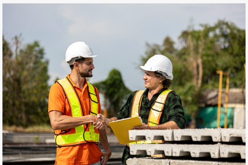
Two workers on site speak with a community representative, demonstrating respect, transparency, and accountability during active operations.
