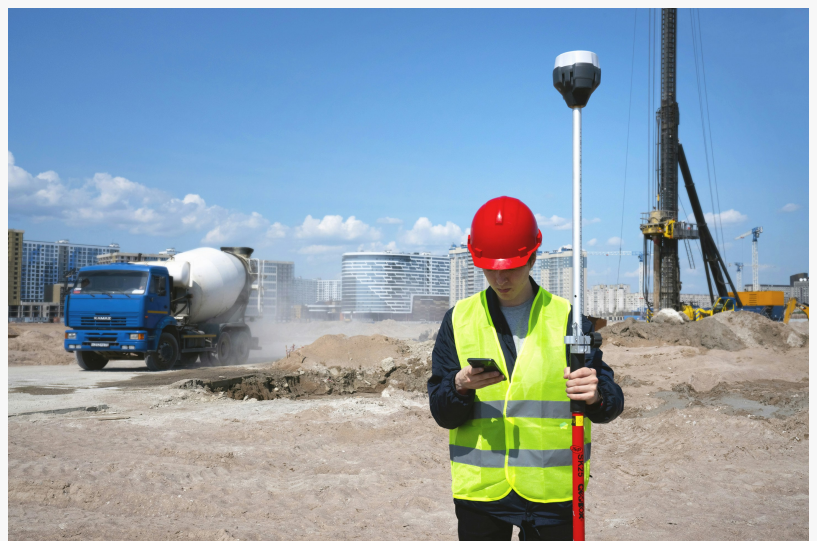
A field manager reviews safety conditions and documentation on an active worksite, ensuring compliance with site inspection and OSHA standards.
