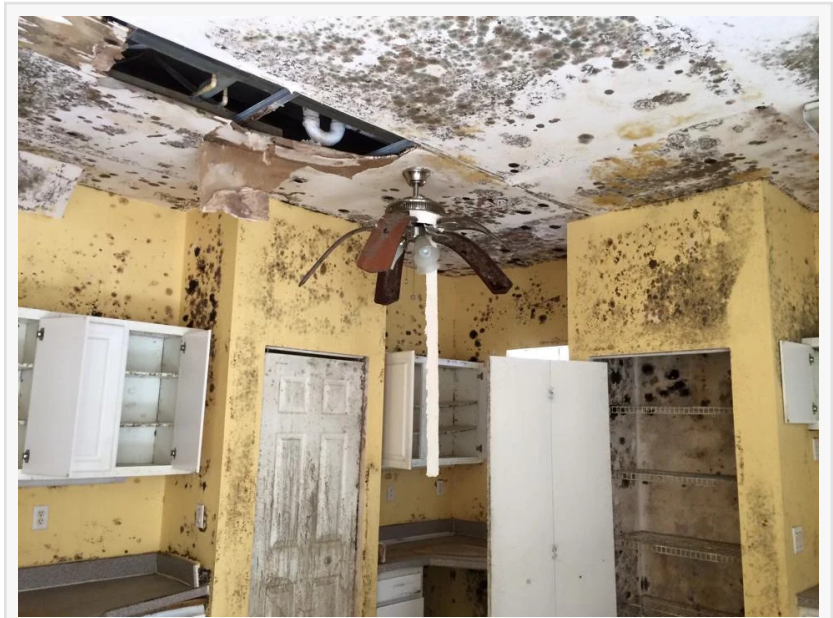
Visible mold growth inside a property after moisture intrusion and water damage, highlighting the need for professional mold remediation.
