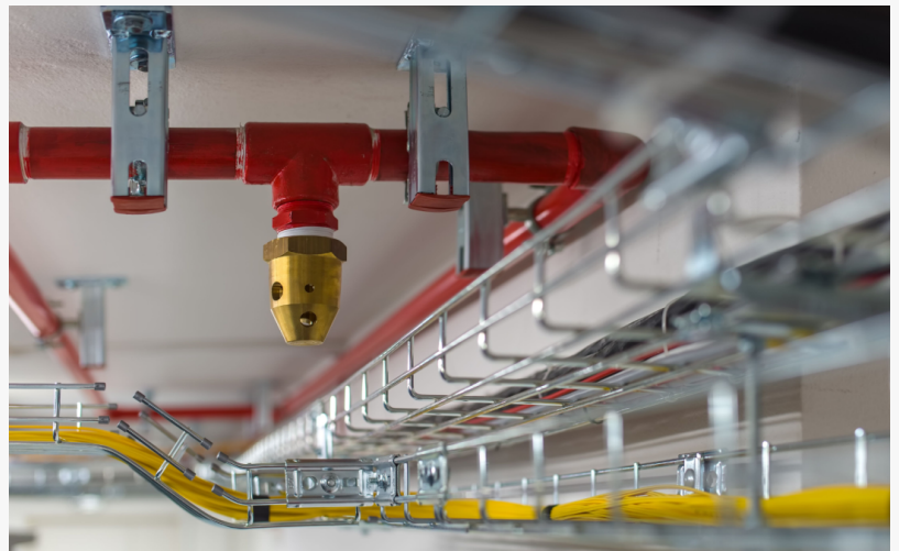
clean agent system close up
