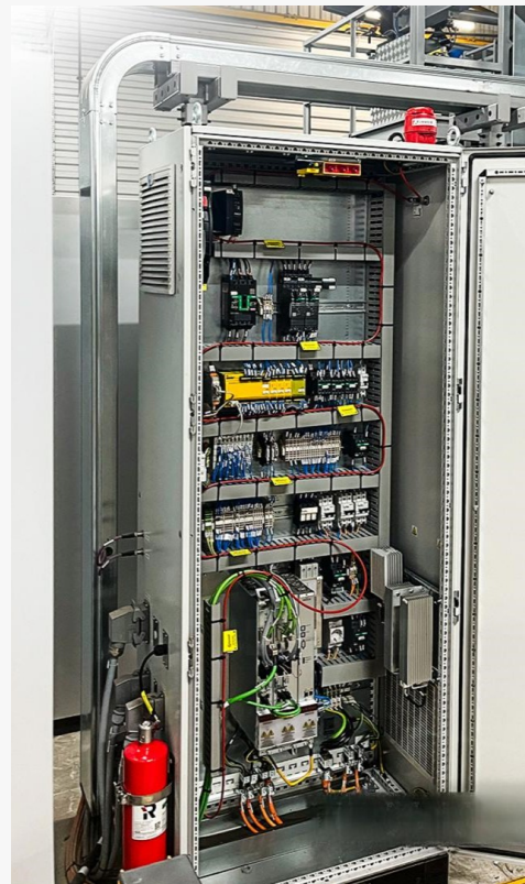
Fire extinguisher electrical
