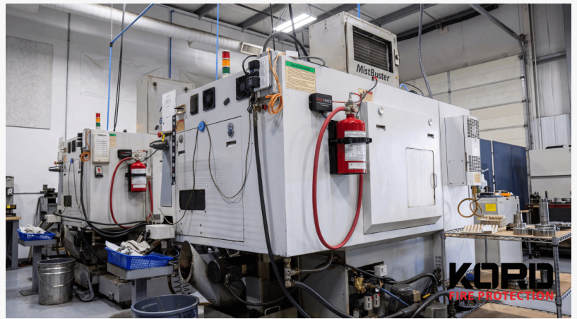
Machinery Fire Systems
