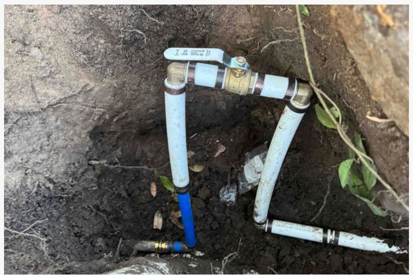
Rerouting provides a new pipe pathway and avoids cutting into Garland foundations.
