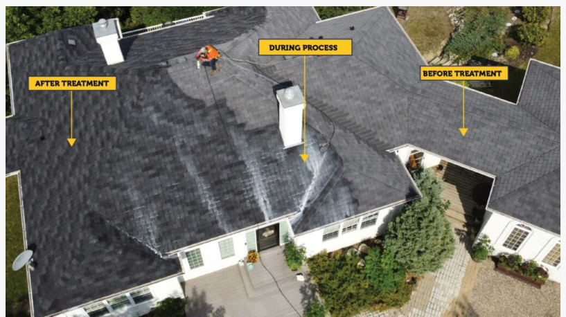
Aerial before, during, and after view of a shingle roof rejuvenation treatment by Tip Top Roofing Service in Scottsdale, AZ. ROC #355034.
