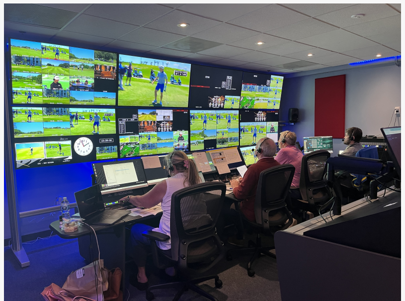
BMG Broadcast Control Room from the NOC
