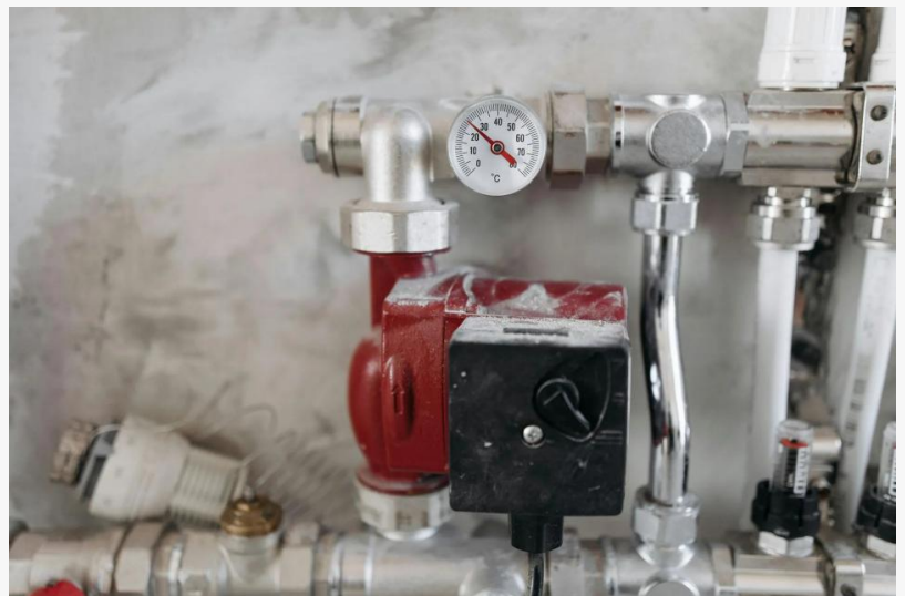
emergency hvac service
