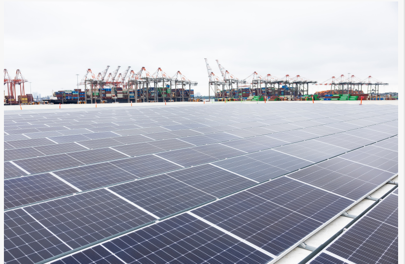
The installation will generate approximately 1.6M kWh of clean energy annually.
