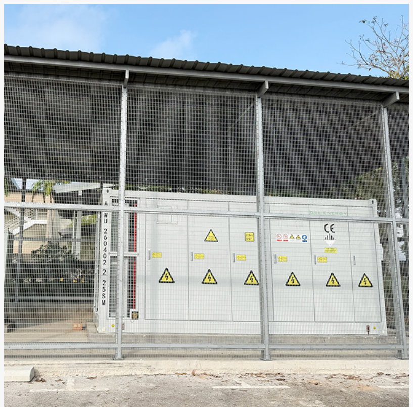
20-foot liquid-cooled BESS container with LiFePO4 battery technology for commercial and industrial energy storage applications
