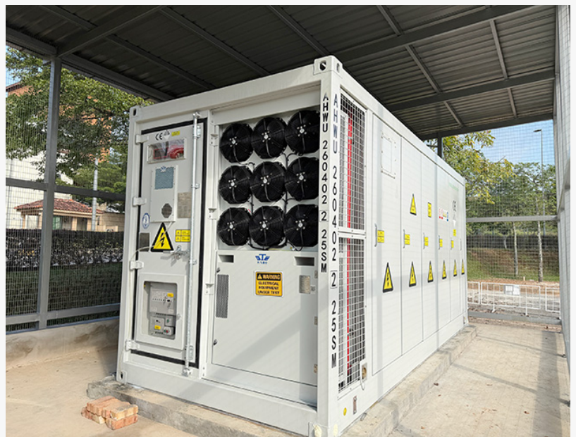
Outdoor commercial battery energy storage system installed beside a shopping mall in Malaysia for intelligent energy management
