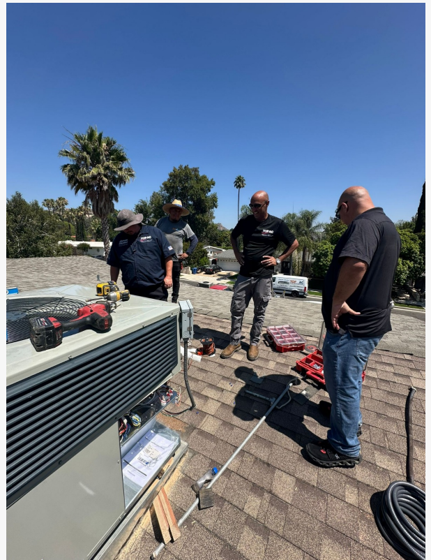
HVAC Contractors Los angeles
