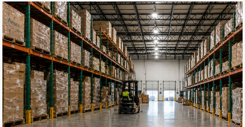
lighting for remodels and contractor jobs
