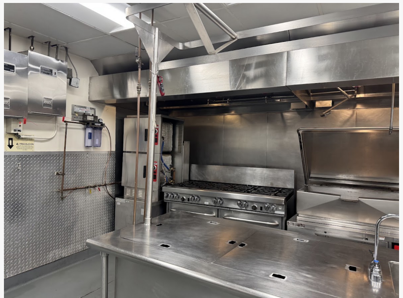
Commercial kitchen after professional deep cleaning and grease removal by CE Kitchen Cleaning
