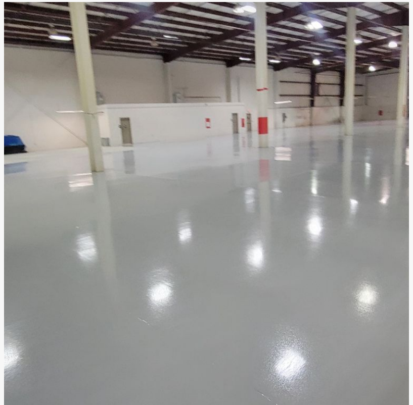
Epoxy Flooring For Warehouses
