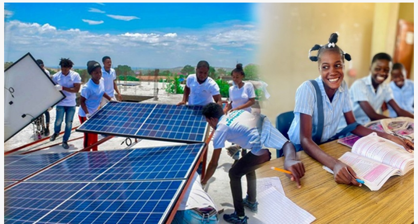
Brighten Haiti Students at a Brighten Haiti Solar4Schools installation where solar electricity powers classrooms, lighting, fans, and computer labs.
