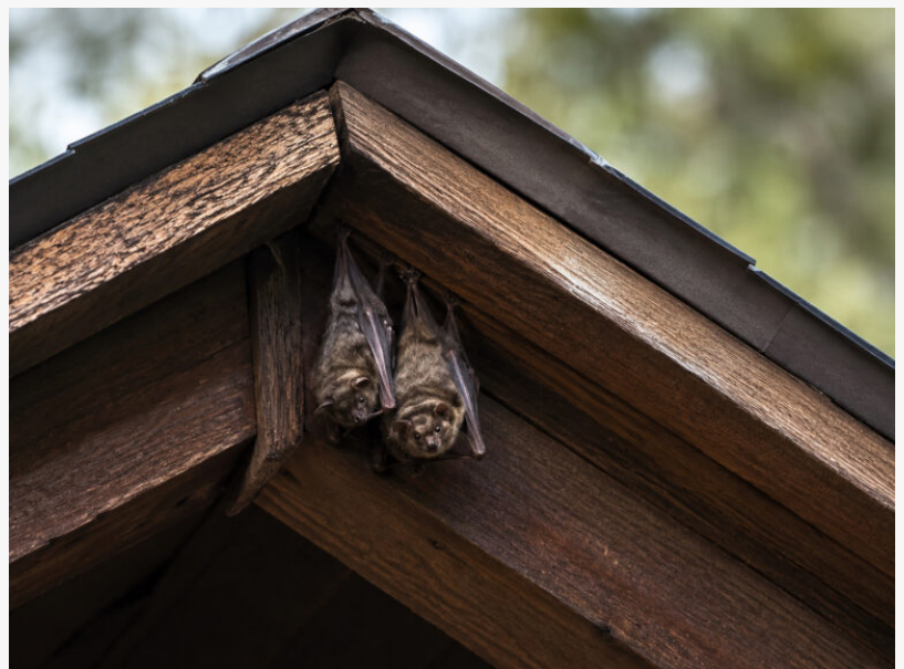
Bats love to find peaks of homes where they can squeeze through openings as small as 3/8"
